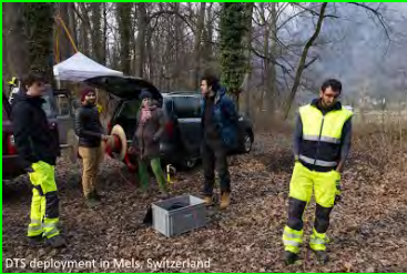
DTS deployment in Mels, Switzerland
