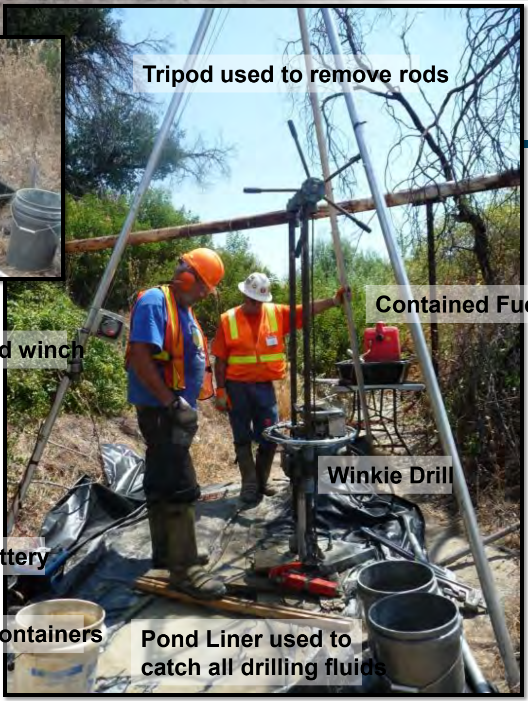
Pump supplies water to drill
